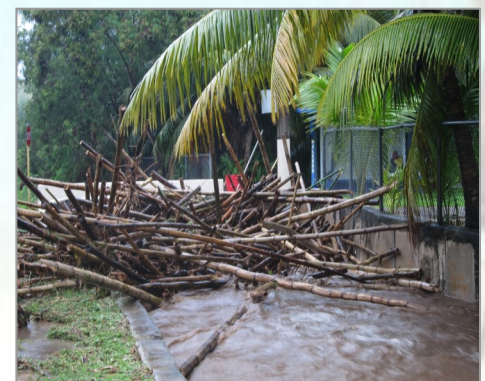
Flood study completed on Manell-Geus watershed. As a result, outreach materials for flood mitigation developed on a residential, governmental and community scale. Site: Flood and bamboo impact on Barcinas culvert (Merizo).
